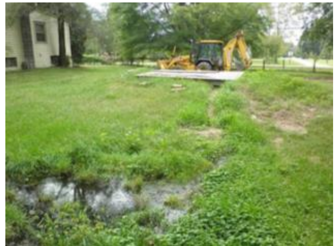
A flooded septic leach field (Cristina Fernandez-Baca)
