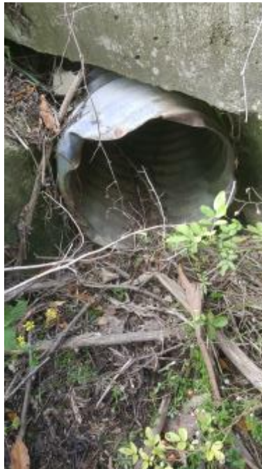
Small culvert in need of maintenance and inspection
