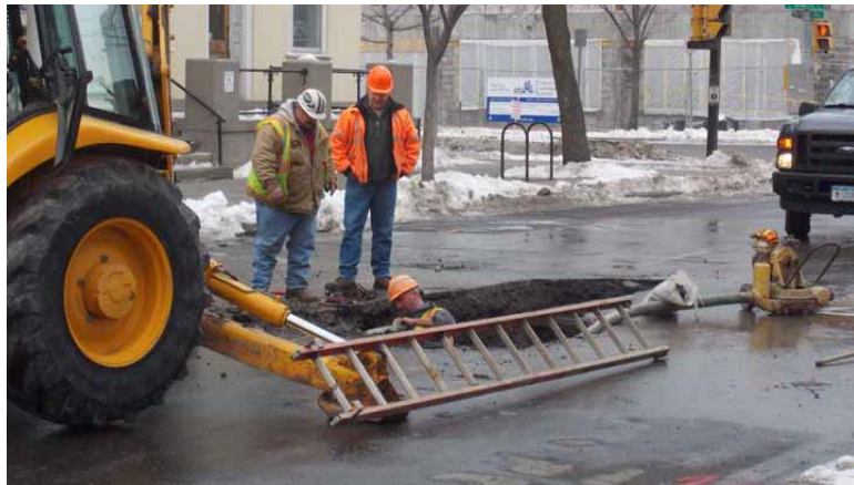
Water main break in Cayuga St, Ithaca (2013)
