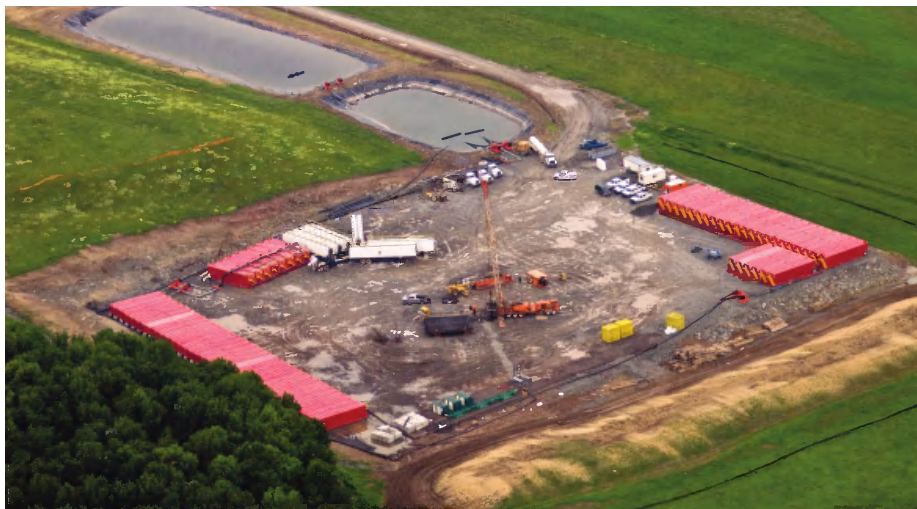
A Marcellus site in Bradford County, Pa. The red tanks hold water.
